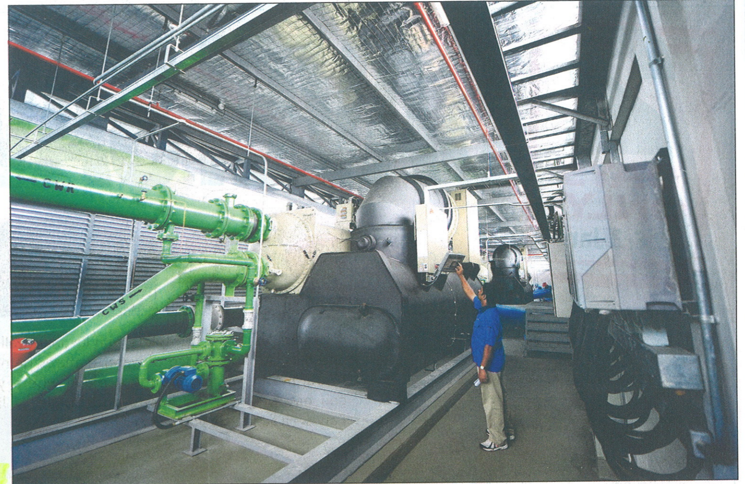
A worker monitoring chillers on the rooftop of Ascendas' headquarters at the Singapore Science Park. The $3.5 million power-saving investment, installed in 2008, is expected to help Ascendas shave $1 million off its yearly utility bill. ST PHOTO: DESMOND LIM
